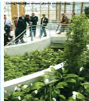
Living machine that cleans black and grey water coming from the buildings
